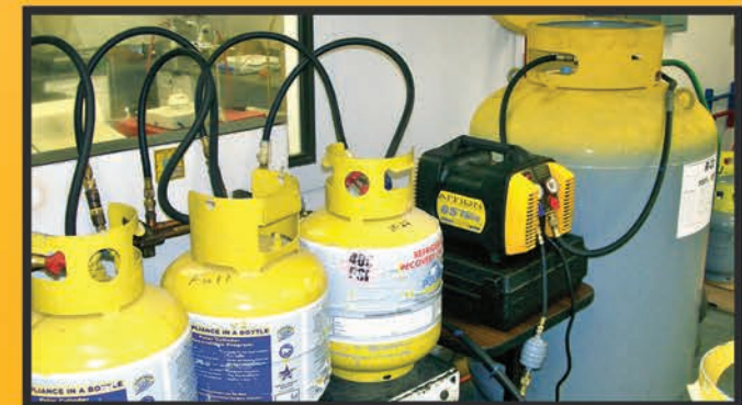
Below: G5Twin used daily in reclamation facility for tank to tank transfers.
